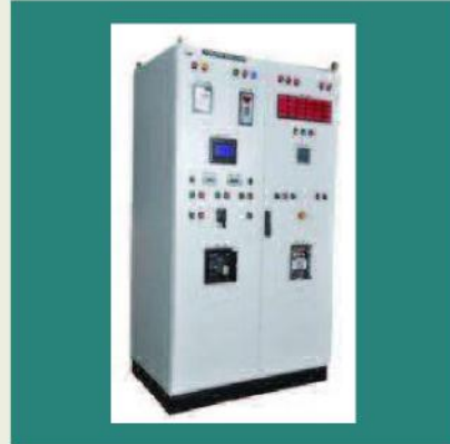
Auto Pump Control Panel
