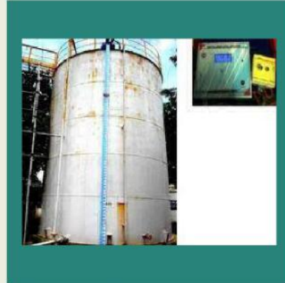
Storage Tank Level Indicators
